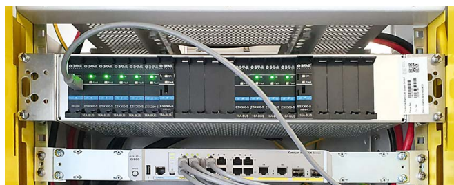
ControlPlex® Rack: protects, controls and monitors the communication systems of the Deutsche Bahn
